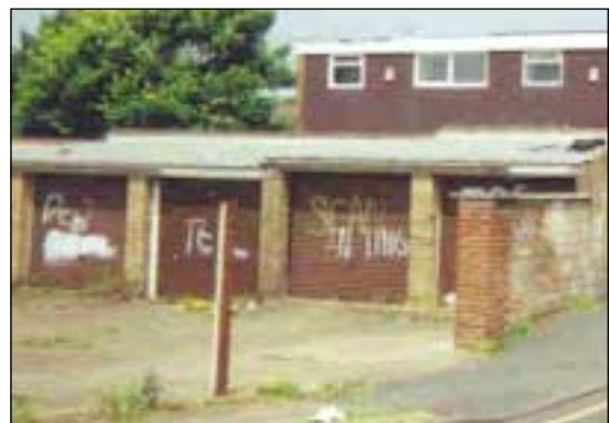
Fig 54: Unlit garage block with poor surveillance becomes a target for crime and vandalism. Source: Northamptonshire Police
